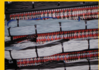
Examples of wiring
