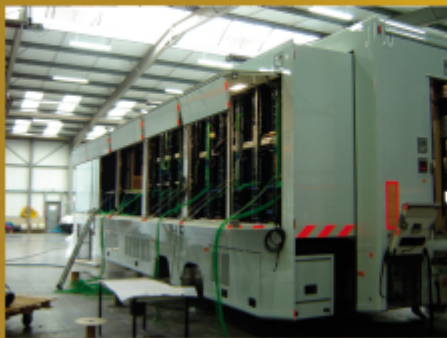
Cable installation in the slideout of an OB Van
